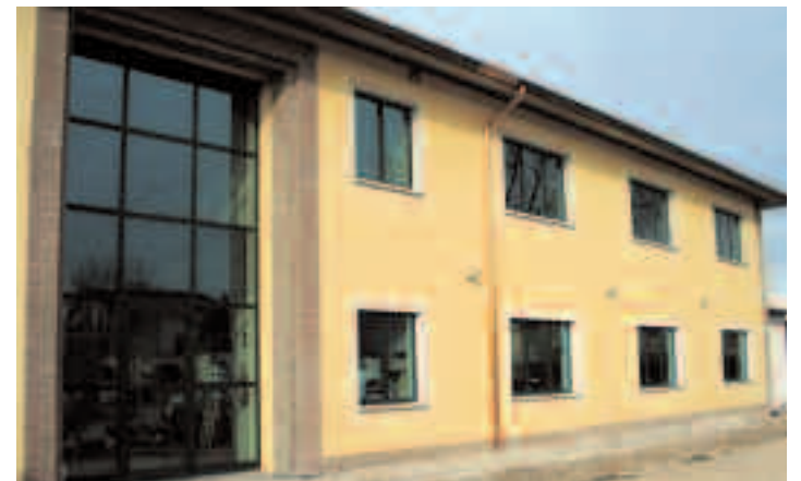
The new building (under construction) has two floors, each with 300 square meters of space, ten times the previous office area.
