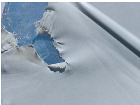
A severe case of coating failure due to improper cure time and temperature.
