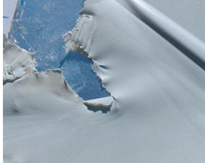
A severe case of coating failure due to improper cure time and temperature.
