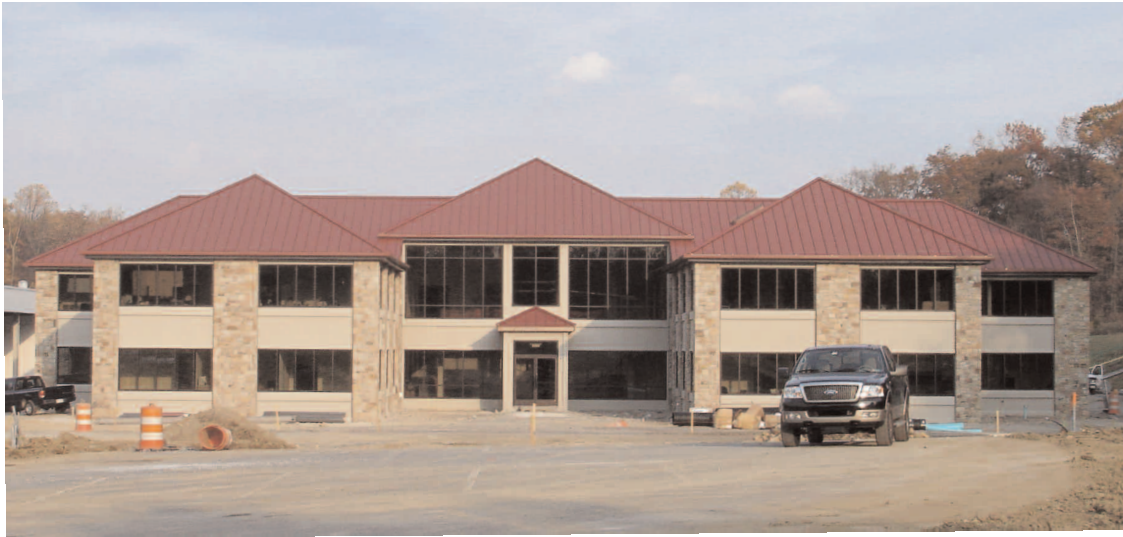
Whitford's new worldwide headquarters (under construction) at the new location in Elverson, Pennsylvania. The office is 23,000 square feet, the factory is 210,000 square feet.
